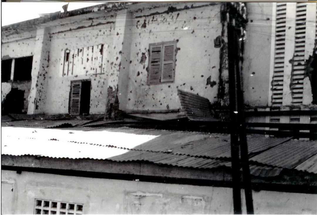
133. "A town called Baria not far from Vung Tau". Damage after a fire fight during the Tet Offensive, 1968 South Vietnam.
